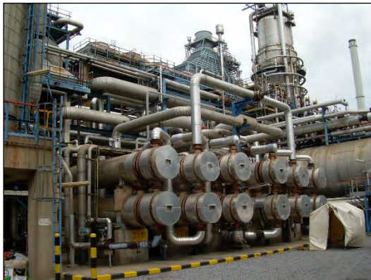
High temperature vibration measurements
